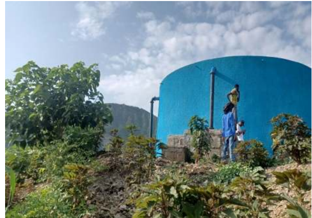
A 500 cubic meter reservoir constructed by Habitat Ethiopia and partial view of trees planted to protect the water source
