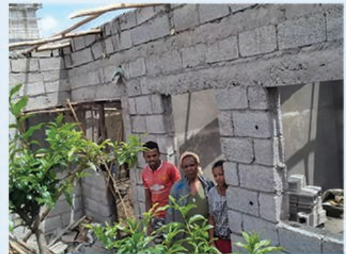
Habitat started construction of house for Yeshareg's family but the pace of work was slow.
